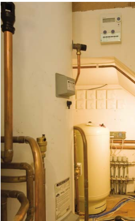
Behind the scenes – The Hometronic Manager lives in the plant room with the boiler, hot water cylinder and underfloor heating manifold
